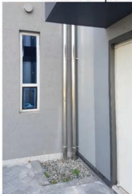
Infiltration by rainwater down spout (Incheon)
