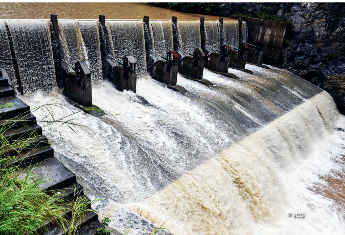
Figure 5-6 Chongqing City: A small hydropower in the aftermath of a flash flood event; Green small hydropower can ensure ecological flows of rivers and bring vitality to economic development
